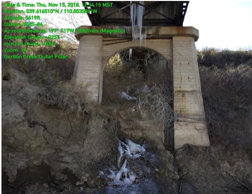
Figure 11. Gordon Creek flume south pier showing stream channel erosion
