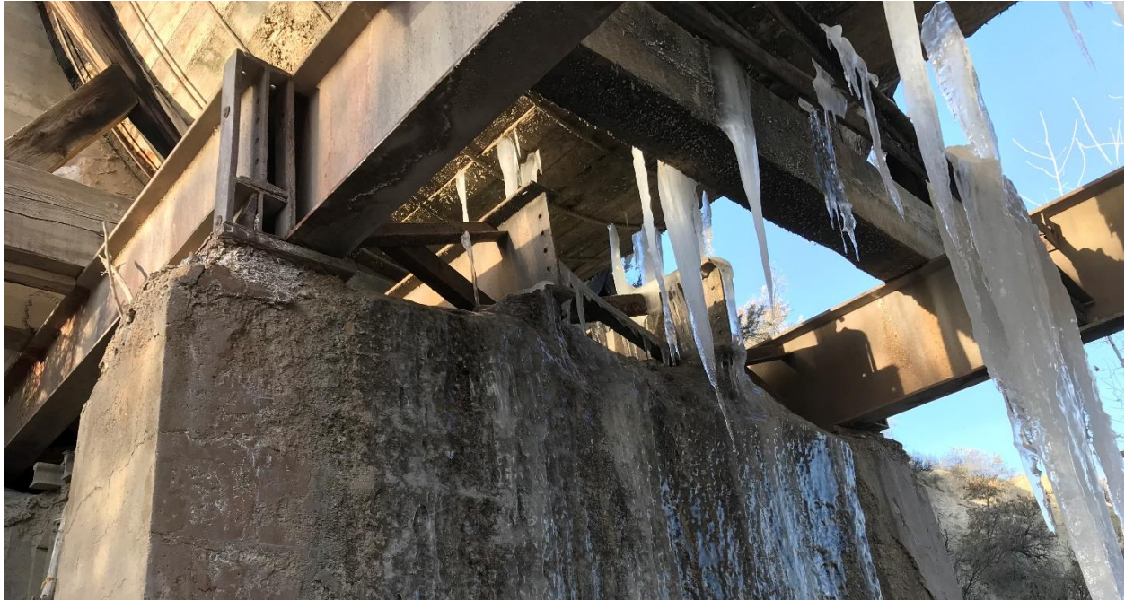
Figure 21. Miller Creek flume south pier showing concrete erosion
