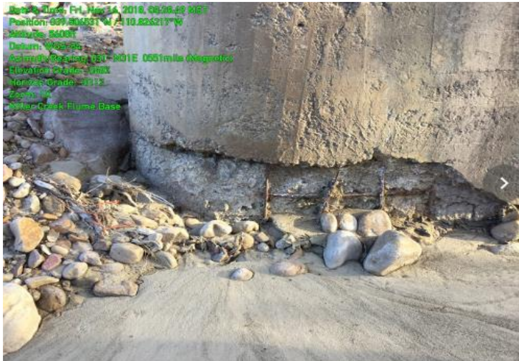
Figure 22. Miller Creek flume center pier with exposed and corroded rebar
